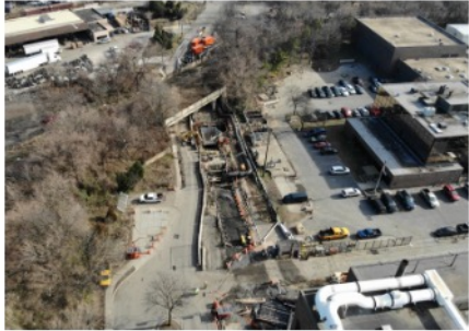
Separation of the combined stormwater and sanitary sewer systems in Pennsauken Township.
